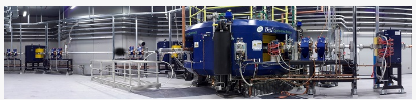
Best 70 MeV Proton Cyclotron installed in INFN, Legnaro, Italy (Photo courtesy of Laboratori Nazionali di Legnaro)
